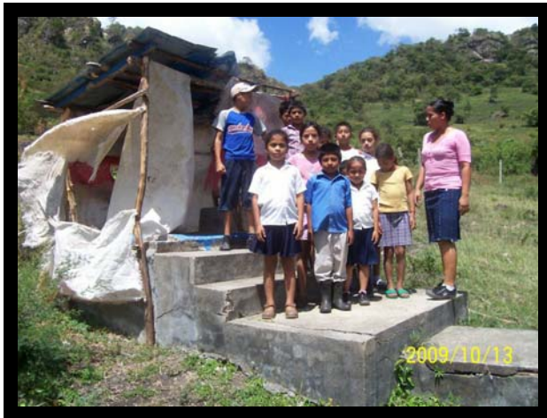
Before: School latrines at Tempisque School
