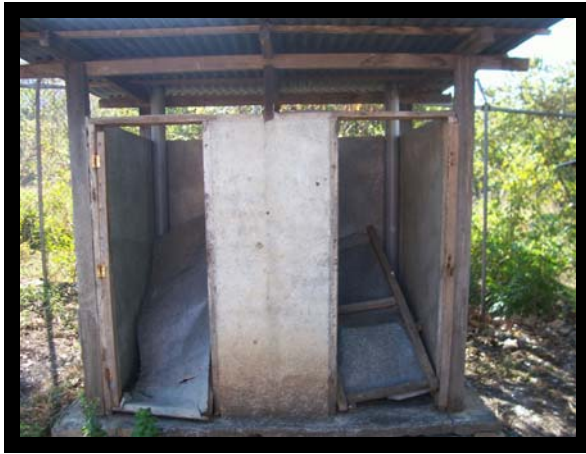
Before: Deteriorated Latrines at Andres Castro School
