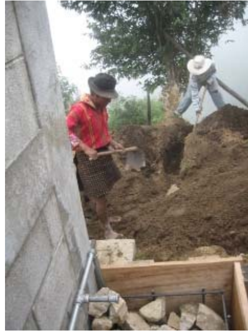
Members of the School Board work on the tube drainage system of the 8-faucet hand washing station.
